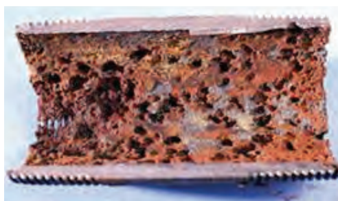
Figure 9.2.12. Condensate pipe – oxygen pitting
