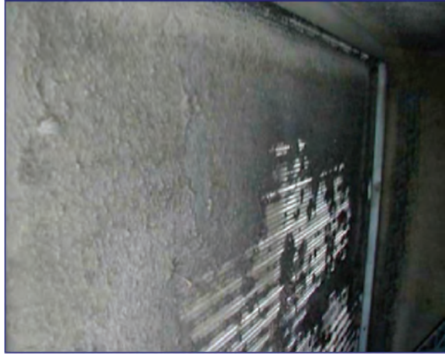
Figure 9.7.1. Cooling coil requiring cleaning
