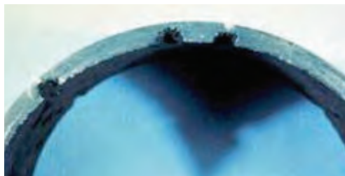
Figure 9.2.10. Feed-water pipe – oxygen pitting
